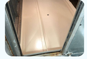
maintenance air treatment unit
