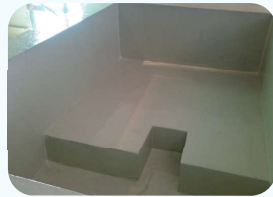
secondary containment protection
