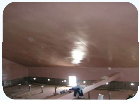
FGD ducts lining
