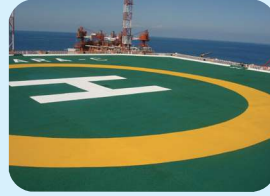
anti-skid helideck flooring
