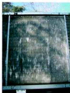
Uncoated fouled and corroded units.
