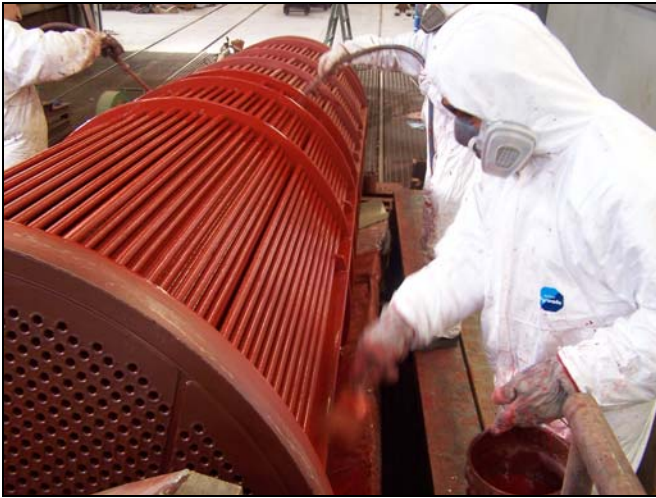
Shell side lining of shell-tube heat exchanger.
