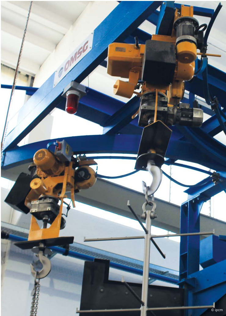
The shot blasting plant is equipped with two hoists.
