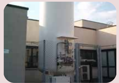
maintenance of technical gases tanks
